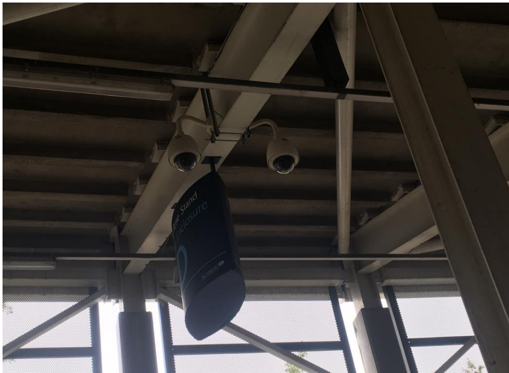
Figure 44 Dome cameras to observe density and flow
