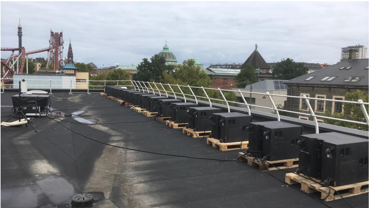
Figure 48 Subwoofers Subwoofers on the roof of the Concerthall – trying to stop the unwanted noise
